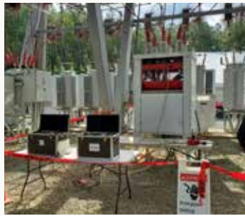
Switchgear and Circuit Breakers
