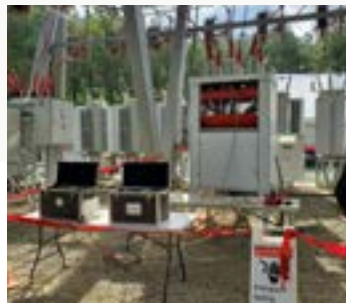
Switchgear and Circuit Breakers
